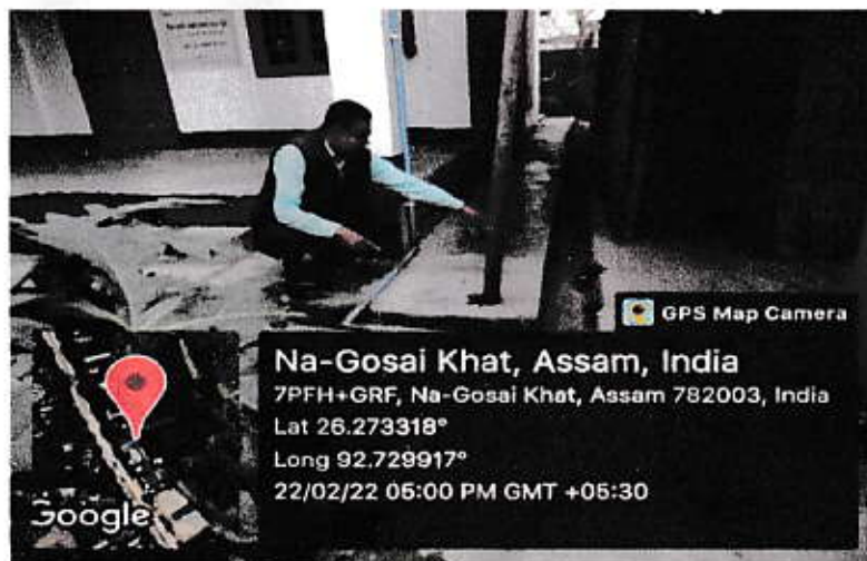
Rain water Harvesting
